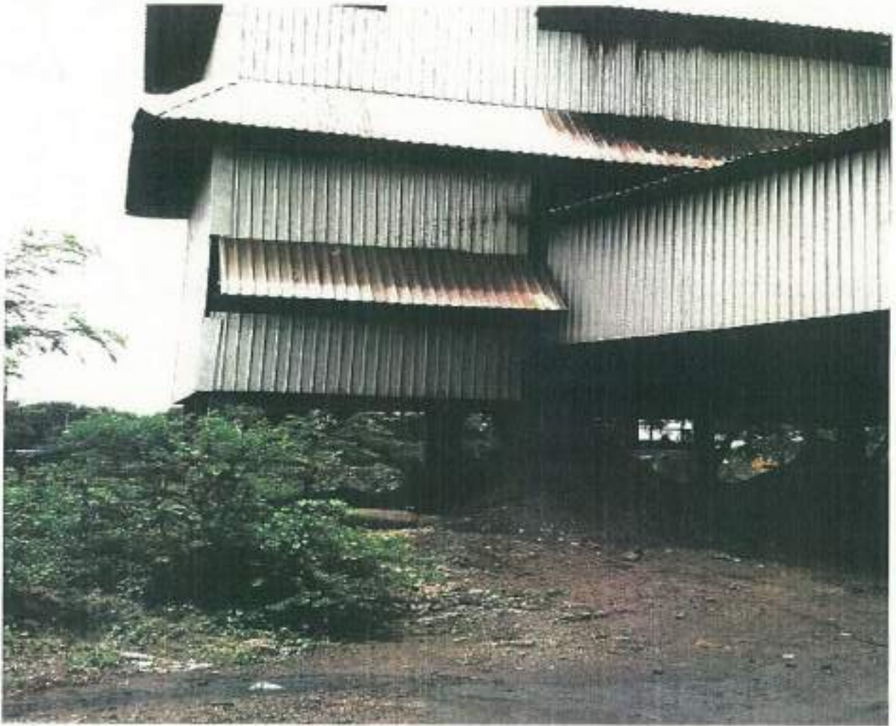
Conveyer Belt transfer point
